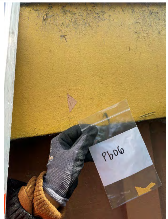
Photo #12: Yellow paint on wood eave, west side of equipment shed.
