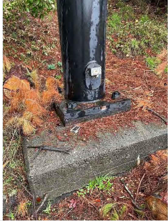
Photo #2: High mast lighting sitting on concrete base, material 101.
